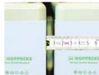
Fig. 5-14: 10 mm clearance between the batteries
