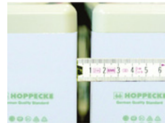
Fig. 5-14: 10 mm clearance between the batteries
